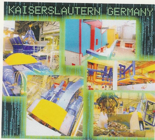
The state-of-the-art plants can be found in municipalities throughout Europe, including Kaiserslautern in Germany
